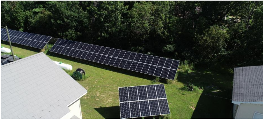
Ho-Chunk HHCD Indian Heights ICDBG Solar Project Photo courtesy Ho-Chunk Housing and Community Development Agency
